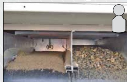
PESATURA INERTI WEIGHING OF AGGREGATES
